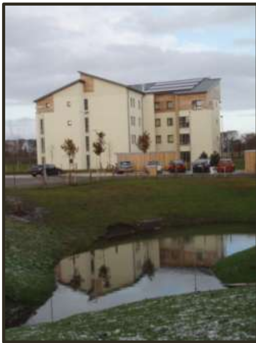
Solar thermal panels at David Russell Apartments
